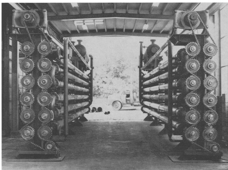
2 Stands of 12 Shells Each, 6" Inner Pipe, All Steel, Drive Cabinet Removed. De-waxing Lube Oils.
